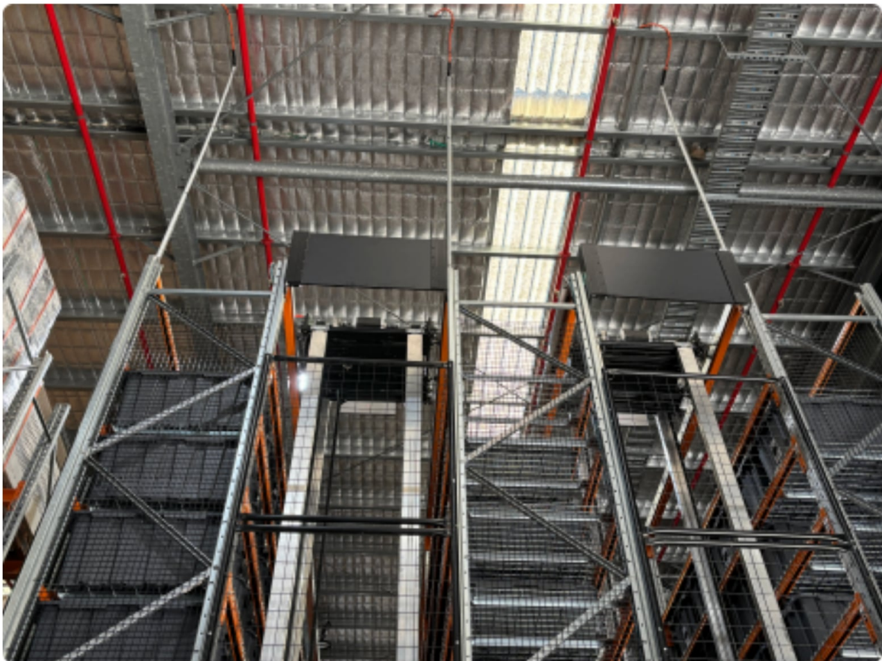
Figure: Example installation with three rows of racking and two Shelfbots
